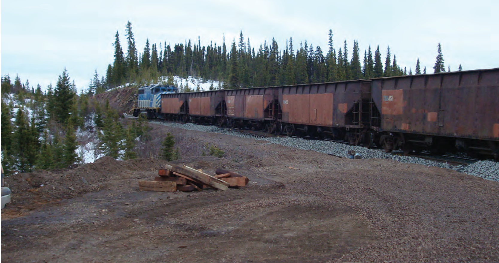
Above - top: Construction of new spur line Above - bottom: Loco and rail cars on new spur line Opposite: View towards Schefferville from Houston deposit
